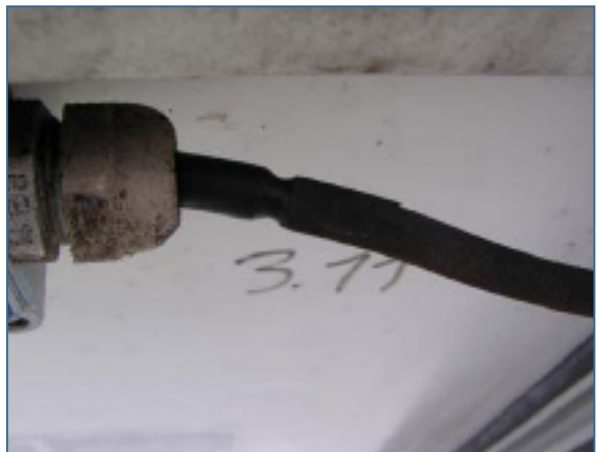
Installation misuse - violent pressure
