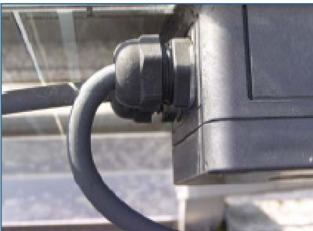
Cable handling misuse - bending radius too small
